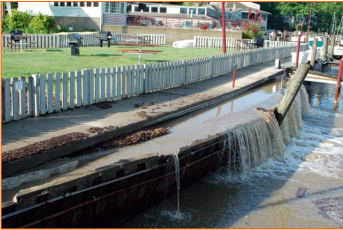
Seawall Damage, June 8, 2008
