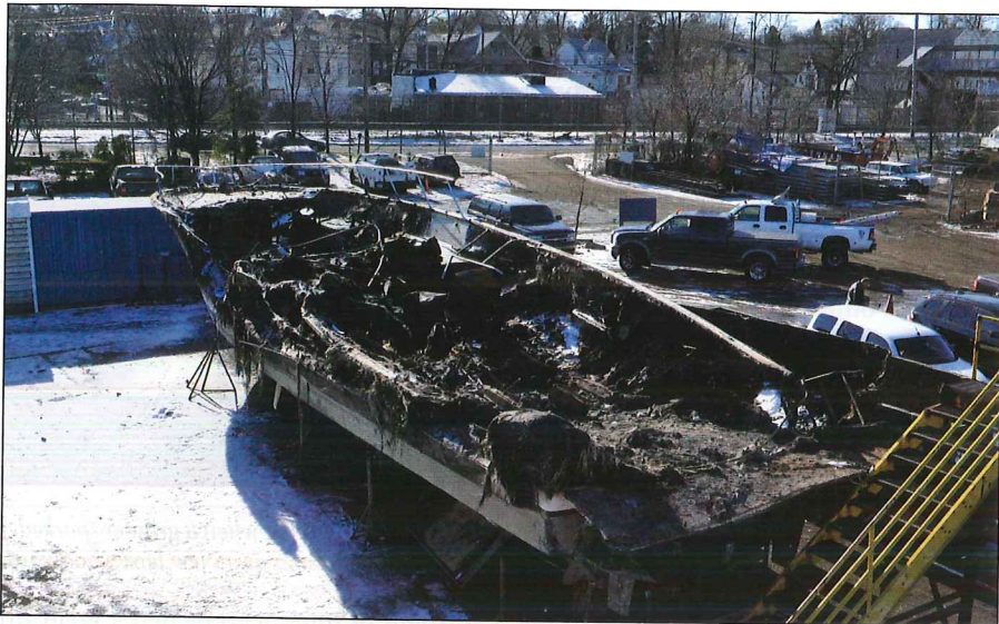
Multiple boats were destroyed in a fire ignited by a heater at Lincoln Harbor Marina in Weehawken, New Jersey.
